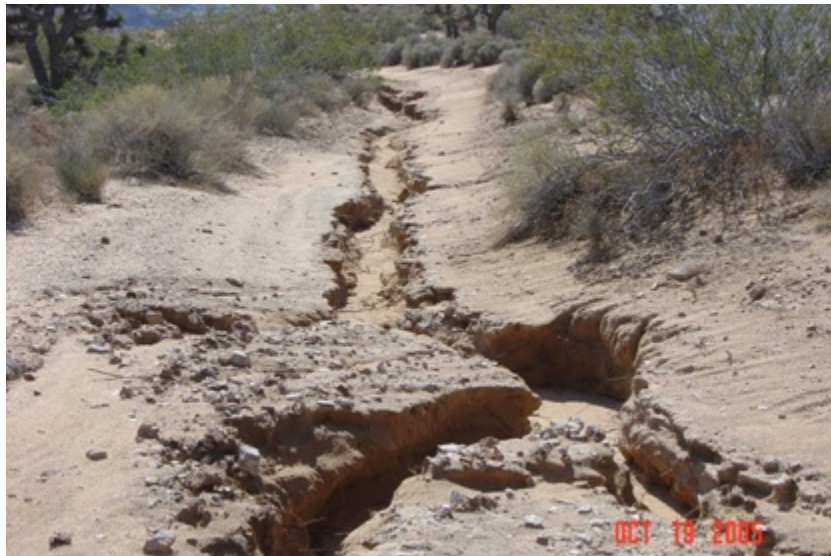
Figure 5. Erosion channels deeply cut into OHV Trail.
